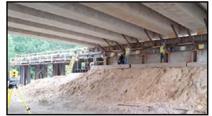
Above, the crew slides the north lanes of the bridge in August. Click here for an MDOT video of the August slide-in.
