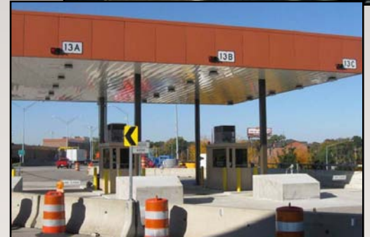
At top, a booth is moved into place. Bottom, the constructed canopy area.
