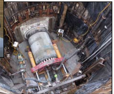
Above, the Genesee County Drain Commissioner's Lake Huron water supply intake project near Port Huron, MI was chosen by the American Council of Engineering Companies of Michigan for an Engineering Merit Award and by the American Public Works Association-Michigan Chapter for a Public Works Project of the Year Award in the Environment, $25M+ Category.
