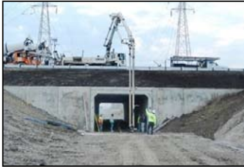
Concrete sidewalk was placed on the inside of the culvert for the future multi-use path.
