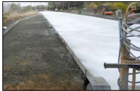
Martin J. Concrete utilized a concrete paver to place the four outside lanes of pavement on the five-lane-wide concrete roadway; the center lane was hand-paved.
