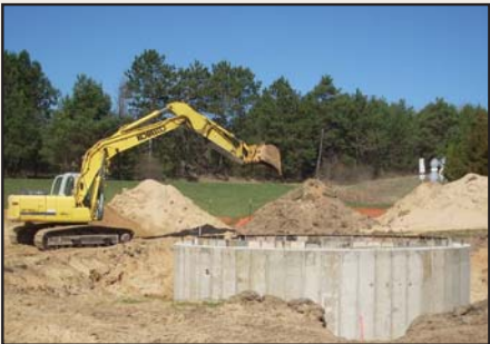
Work on this project in the City of Gladwin costs less due to low bids and 40 percent forgiveness on a DWRP loan.
